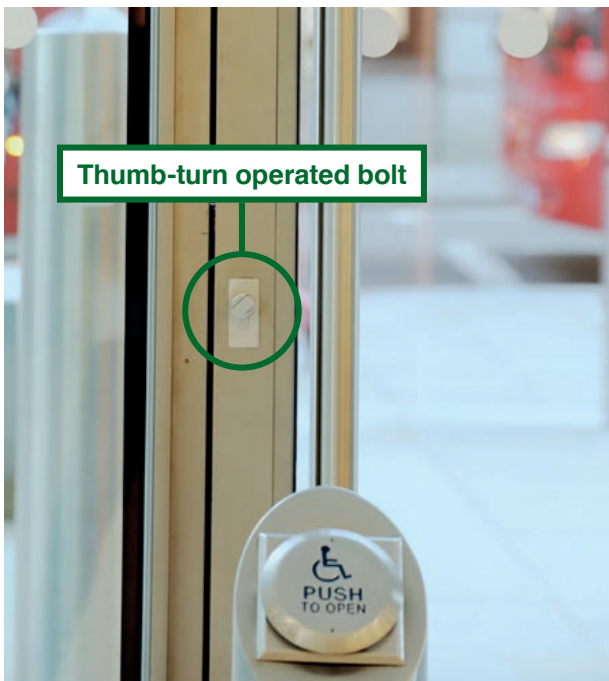
Figure 8: Thumb-turn operated secondary door bolt fitted to an external door constructed with framed glazing
